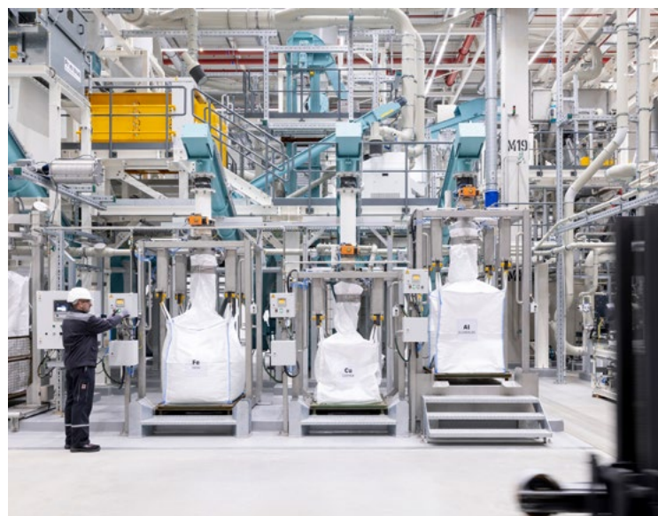
Technology from NRW: Primobius, a subsidiary of plant manufacturer SMS group, handed over a newly built battery recycling factory to Mercedes-Benz in 2024.
